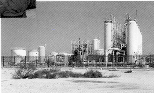
Right photo: The antiscalant dosage is being optimized at this 12 MGD Ras Abu Jajur RO plant in Bahrain.
