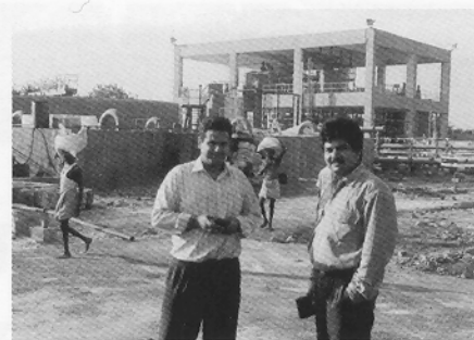
Project engineers at a new RO plant construction site for GMF Power Plant in Chennai (Madras), India.
